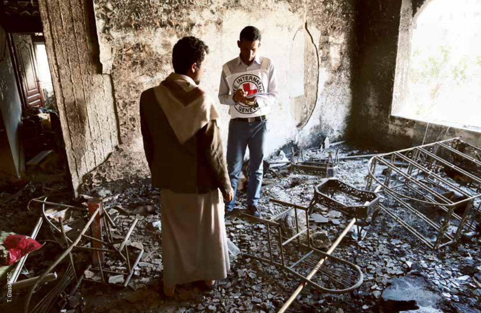
During an evaluation of the damage caused by fighting in the Yemeni city of Sana'a, an ICRC employee listens to a resident describe his situation. April 2015.
