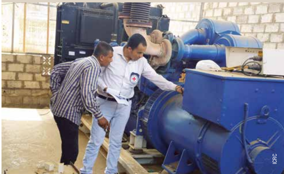
An ICRC engineer checks the motor of a power generator in Hodeida, Al-Thawra Hospital. May 2016.
